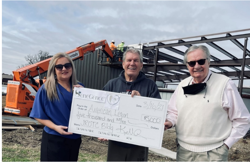
(L to R) Kendra McColloch, Major Jerry Swepston, and Ted Fisher at construction site at Sapulpa High School
